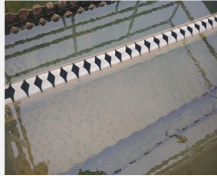
Lamella Clarifier (Broken Lamella : over than 50%)
